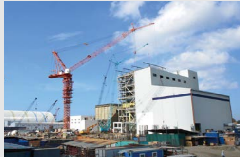
The Puting Bato 2x135MW Coal-Fired Power Plant in the Philippines Project
