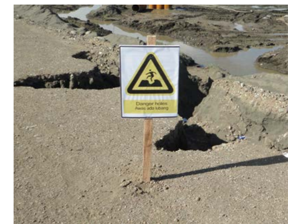
Safety signs for Adipala Power Project
